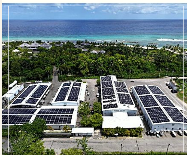
Five rooftops at Heart of House, with the reef line beyond. The system is engineered for coastal corrosion and hurricane-force wind.
